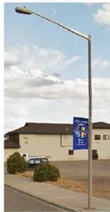
EXISTING STREET LIGHT With banner
