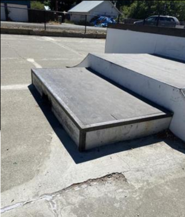
Structurally failing ramps
