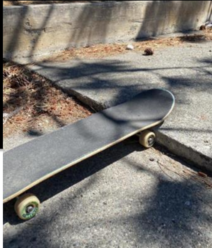
Surface rough, uneven, cracked concrete
