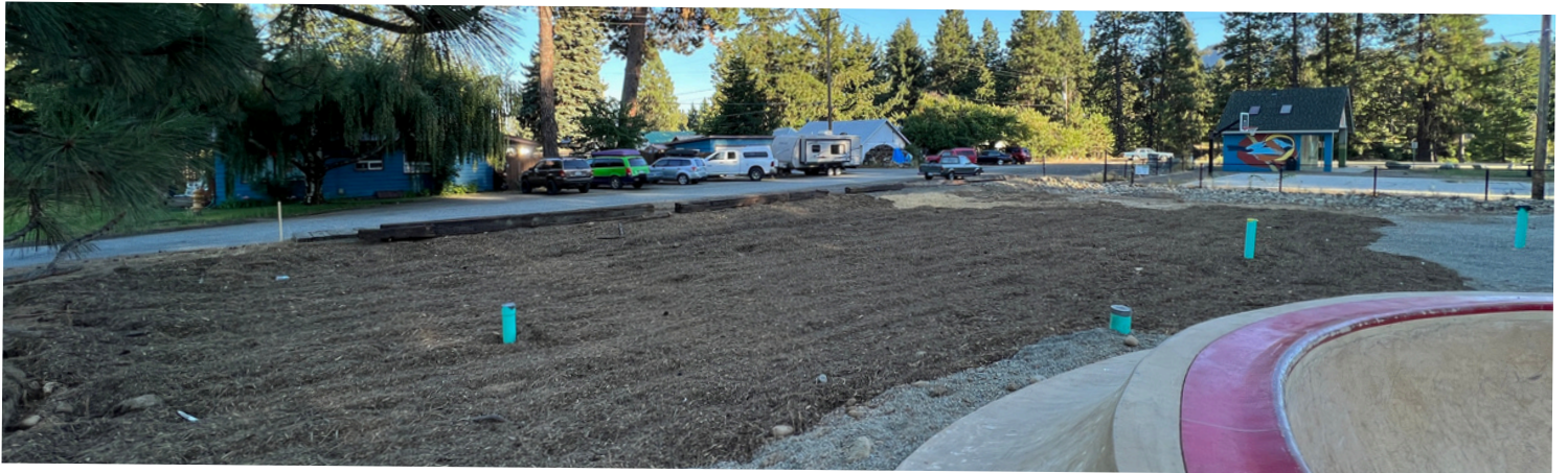
The Phase 2 area mulched with vulnerable in-ground drainage (blue vertical pipes).
