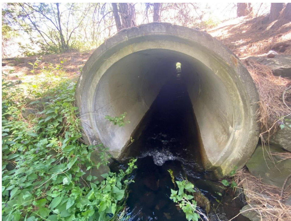
Photograph 5. Inlet of concrete I-90 culvert showing lateral cracking.
